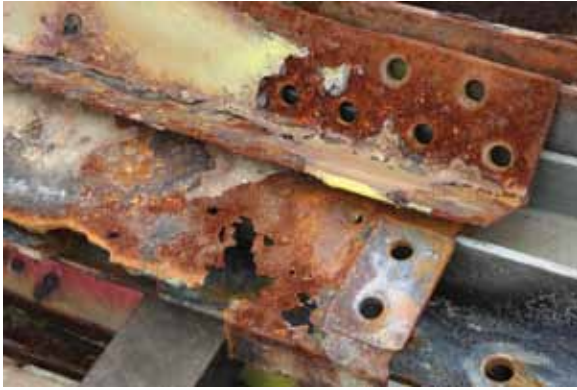
A stack of corroded structural steel members highlights concerns that the dam gates at Montgomery Lock and Dam would not survive a barge strike or heavy ice loads.
