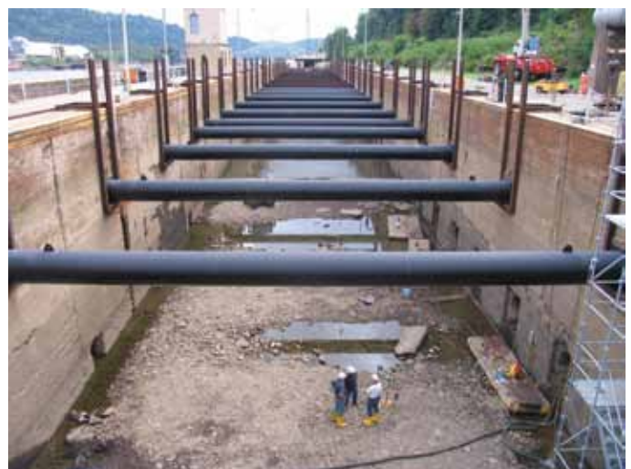
The dewatered main chamber of Monongahela River Lock and Dam 3 at Elizabeth is heavily braced due to its questionable stability. The district has spent more than $7.3 million since 2006 to maintain the locks originally slated for removal in 2004.
